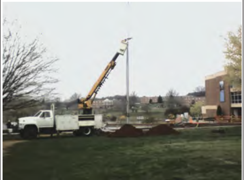
The Hart International Plaza construction crew repositions the flag pole on Monday morning, March 28. photo by Brandon Grimes-Whited
